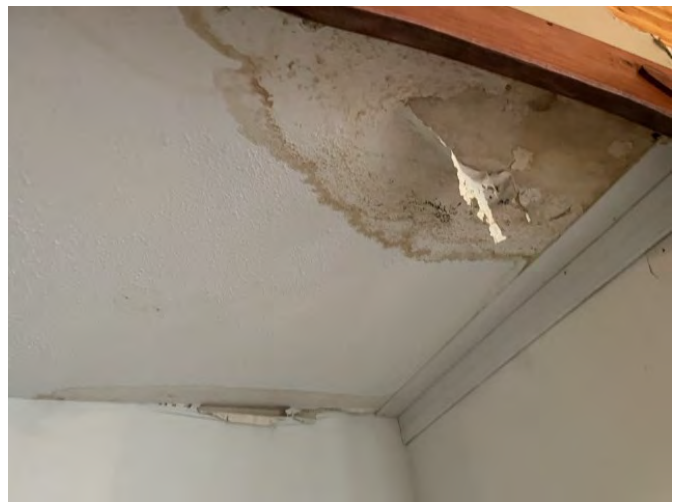
Water damage ceiling of hallway on main (upper) floor.
